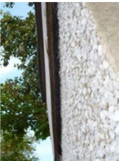
Target Note 7: Electricity sub-station with moderate bat roost potential relating to fascia board gaps.
