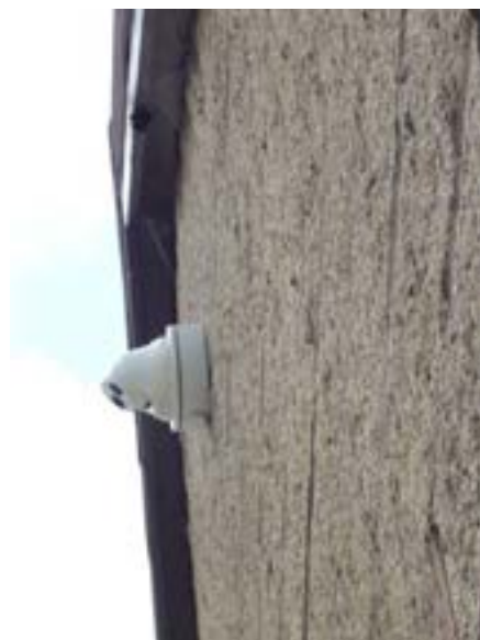
Target Note 6: Clubhouse with moderate bat roost potential; gaps behind fascia's.
