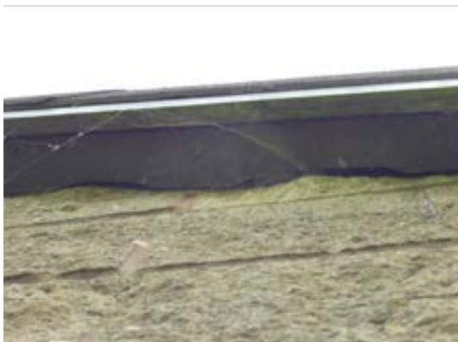
Target Note 6: Clubhouse with moderate bat roost potential; gaps behind fascia's.
