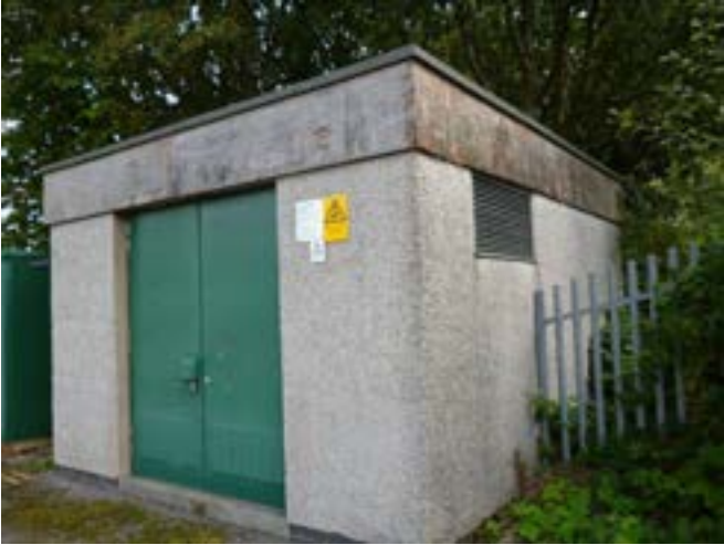
Target Note 7: Electricity sub-station with moderate bat roost potential relating to fascia board gaps.
